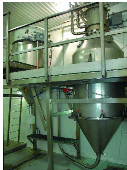
Material dried in this pulse-combustion dryer (right) is collected by a baghouse (left).
