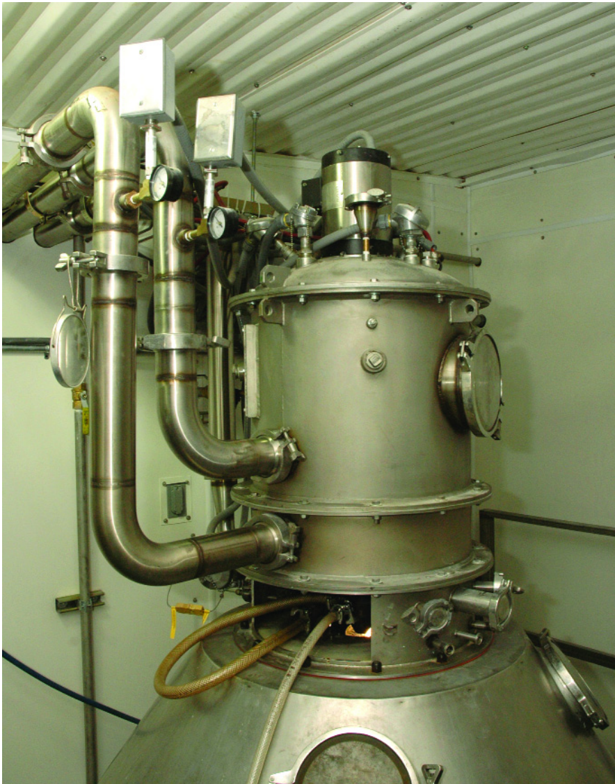
The two large pipes feed quench air (left) and combustion air (right) into the pulse-combustion unit.
